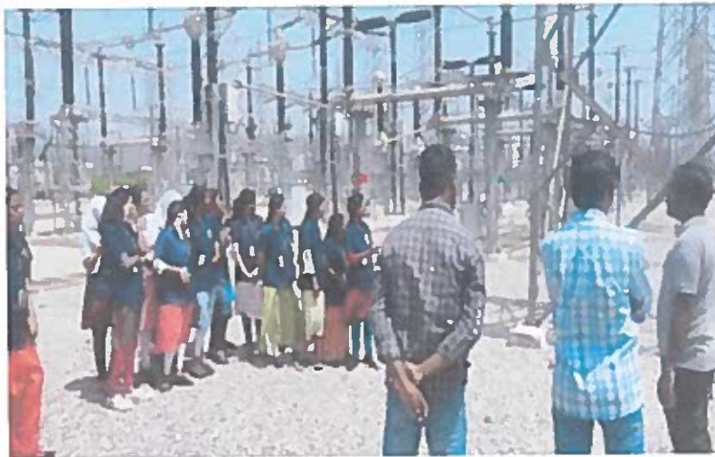
INDUSTRIAL VISIT TO 220/130 KV SUBSTATION
