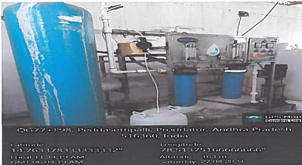
R&O PLANT TO PURIFY WATER FOR DRINKING PURPOSE
