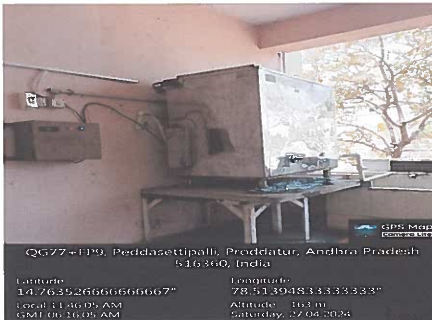
DRINKING WATER FACILITY
