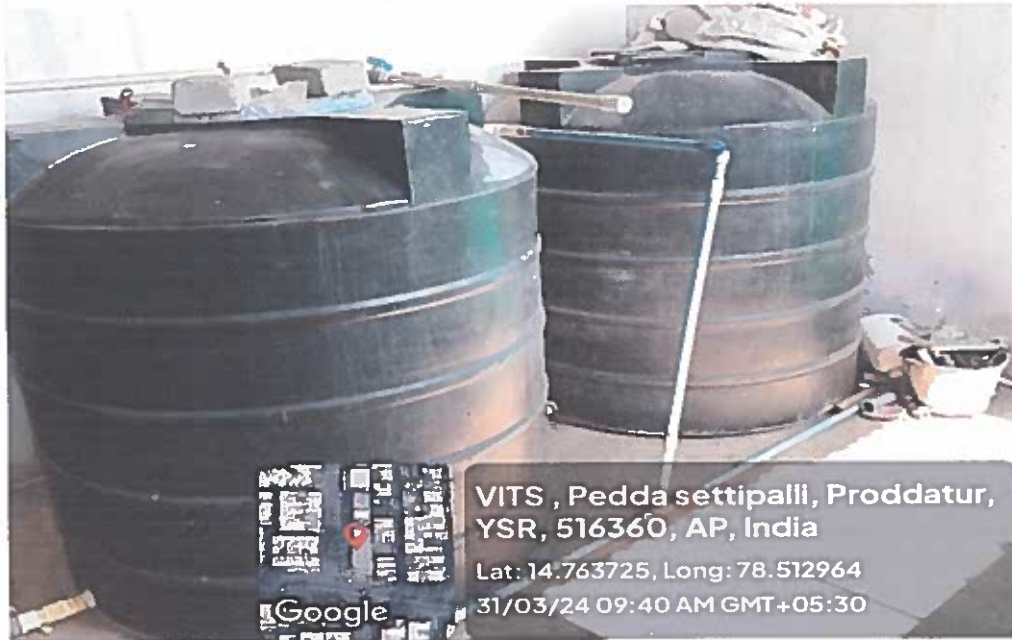
Water Tank at Engineering Main Block with Capacity:2000 Litres
