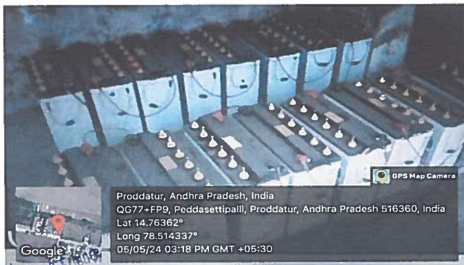
Battery and Inverter Setup
