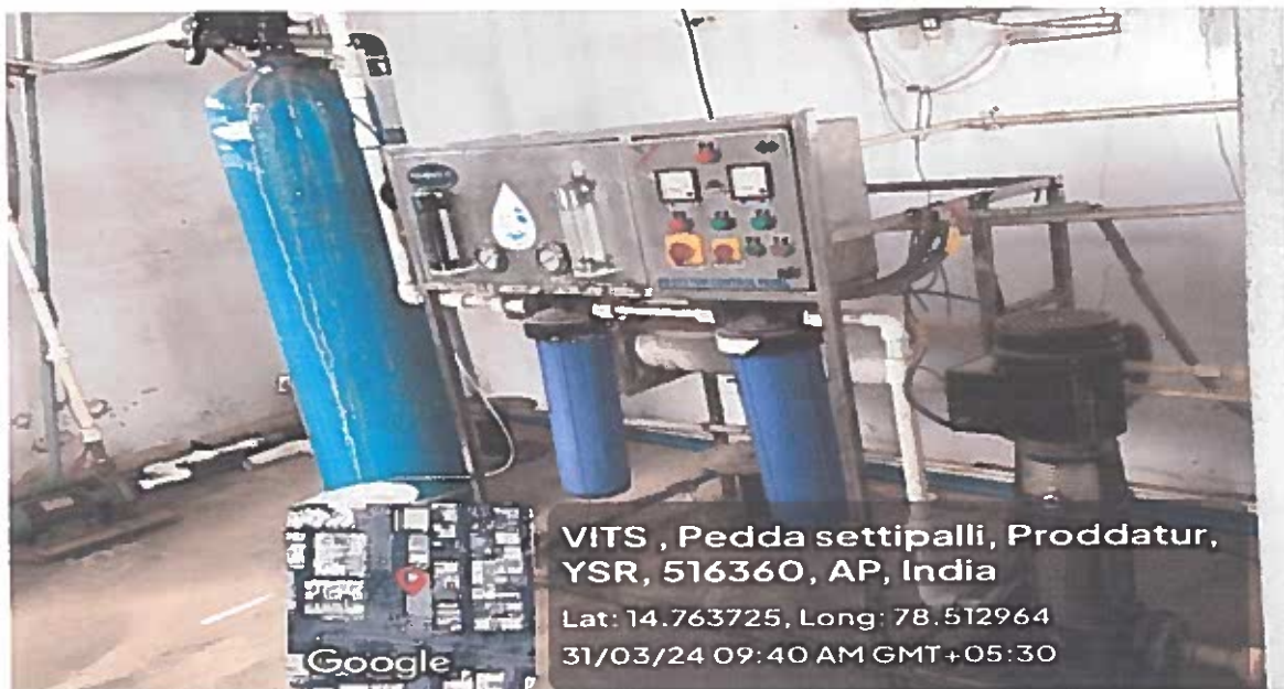
Reverse Osmosis (RO) System at 2nd floor
